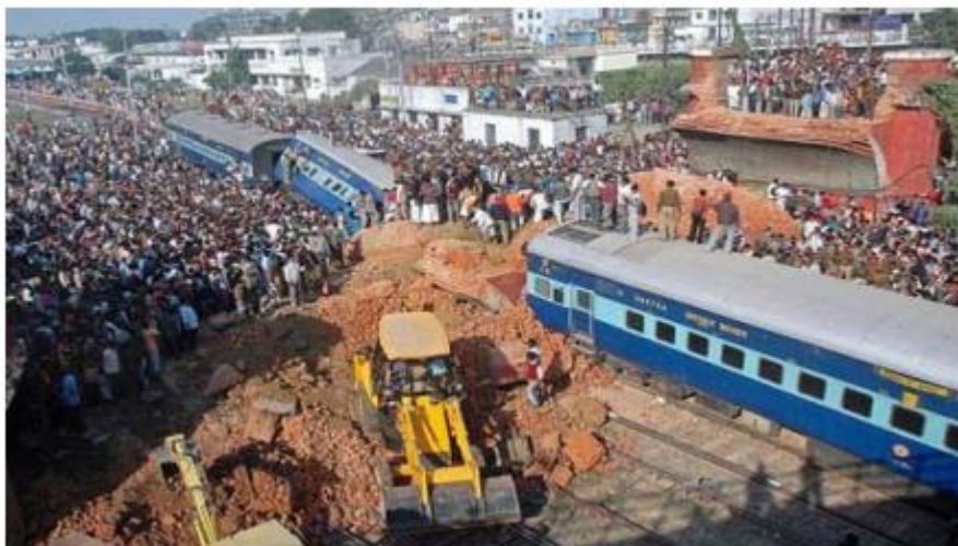
Fig. 1 Collapse of Railway Bridge near Bhagalpur
